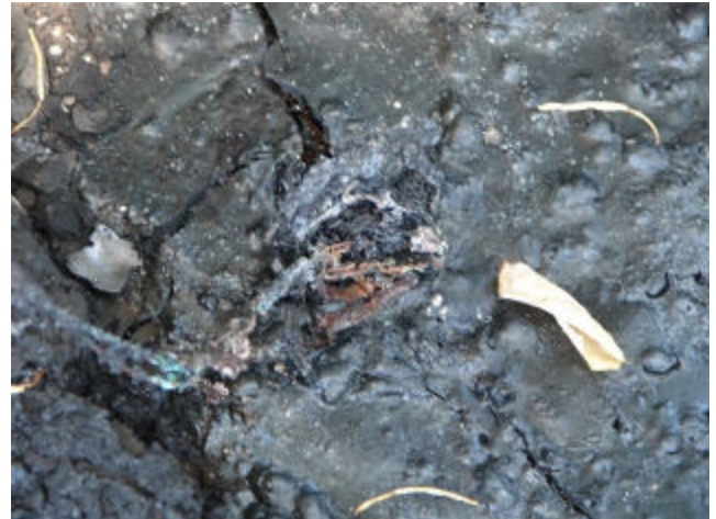
THIS PHOTO SHOWS THE SAVIO UV UNITS BURNED UP WIRES AND LAMP CONNECTION.
